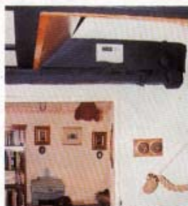
Temperature sensing is by means of CM67 programmable thermostats.
