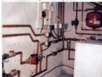
Boiler room at West Mill Cottage, with wiring centre on the left hand wall.
