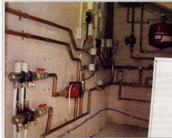
General view of boiler room at West Mill Cottage.
