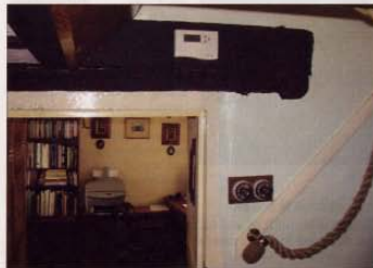
Honeywell CM67 programmable thermostat, mounted in the main hall/stairway.
